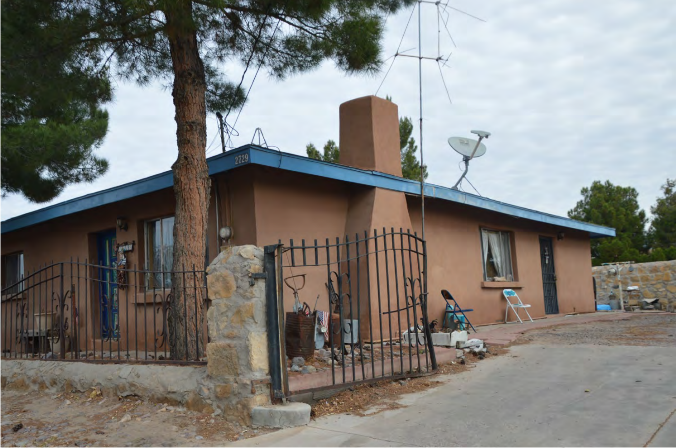
PHOTO FROM CALLE DE SAN ALBINO OF SOUTH SIDE OF STRUCTURE TO BE DEMOLISHED
