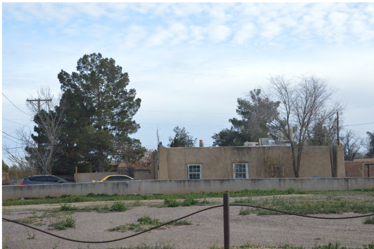
PHOTO OF NORTH SIDE OF DWELLING FROM CALLE DE CORREO SHOWING WINDOW TRIM TO BE PAINTED
