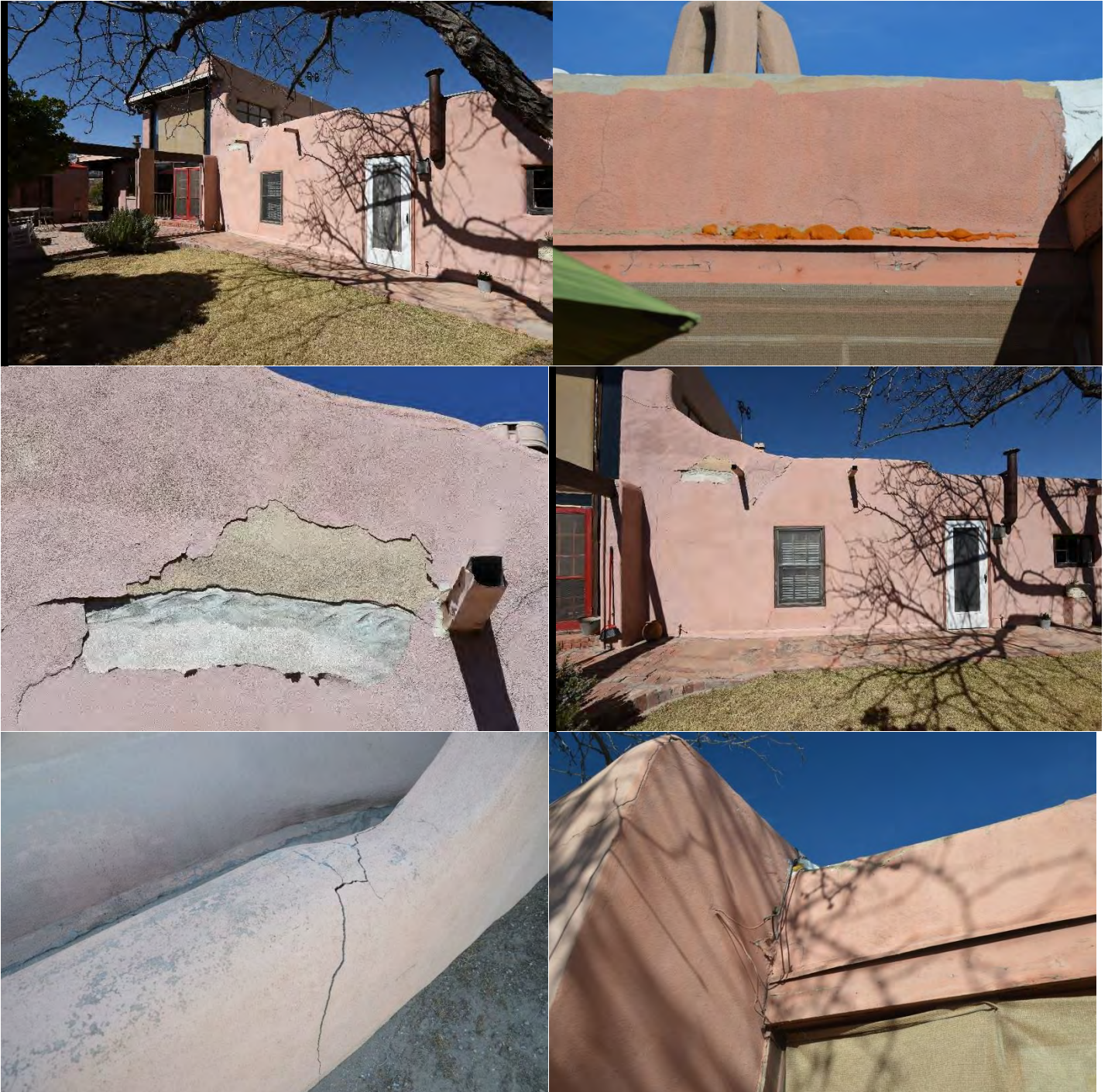
Photos: Examples of widespread exterior plaster issues
