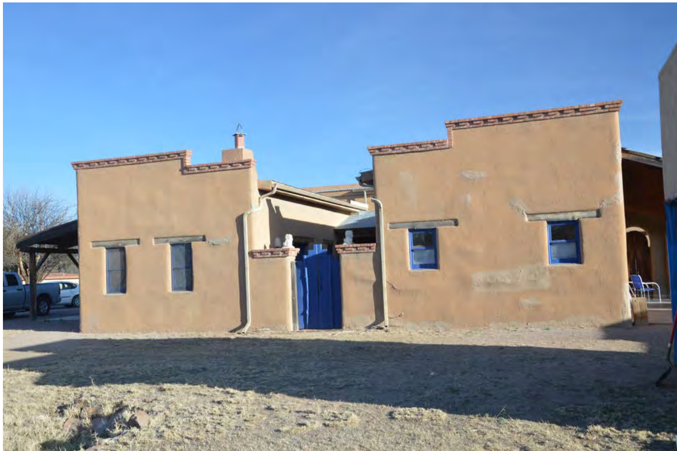
PHOTO OF THE REAR OF THE MAIN DWELLING SHOWING THE EXISTING COLORS
