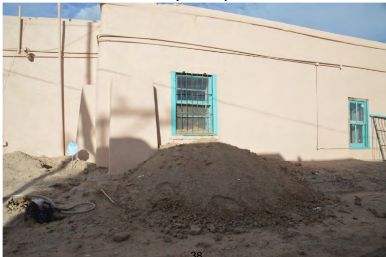
PHOTO OF REAR OF DWELLING SHOWING DIRT (ADOBE) REMOVED FROM INTERIOR (Taken 12/27/18)
