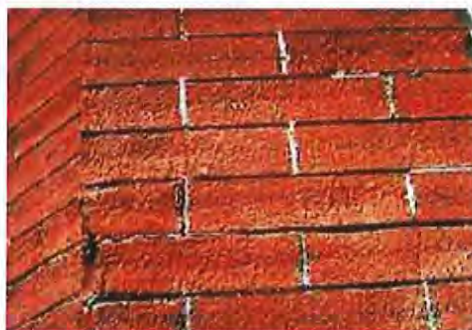
Historic brick damaged by sandblasting.
