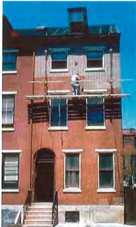
Loss of the historic character due to insensitive repointing.
