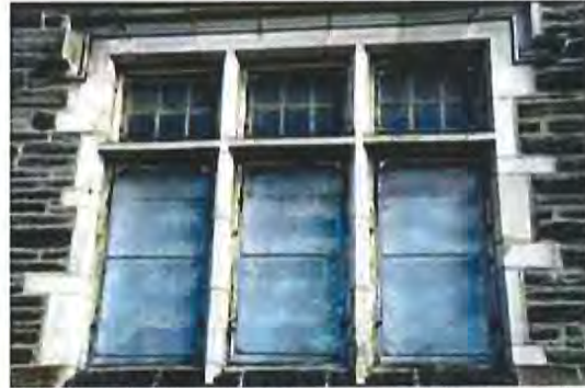
Deteriorated lower window sash shown prior to its replacement in kind.
