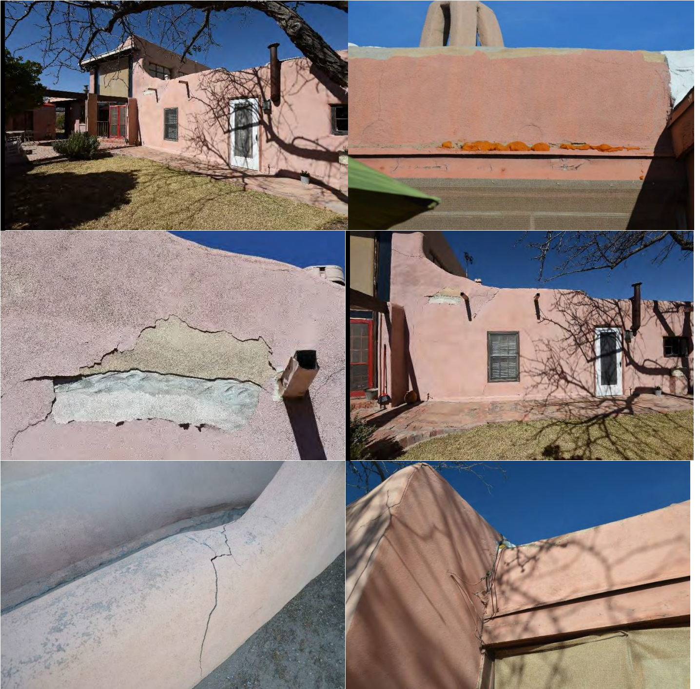
Photos: Examples of widespread exterior plaster issues
