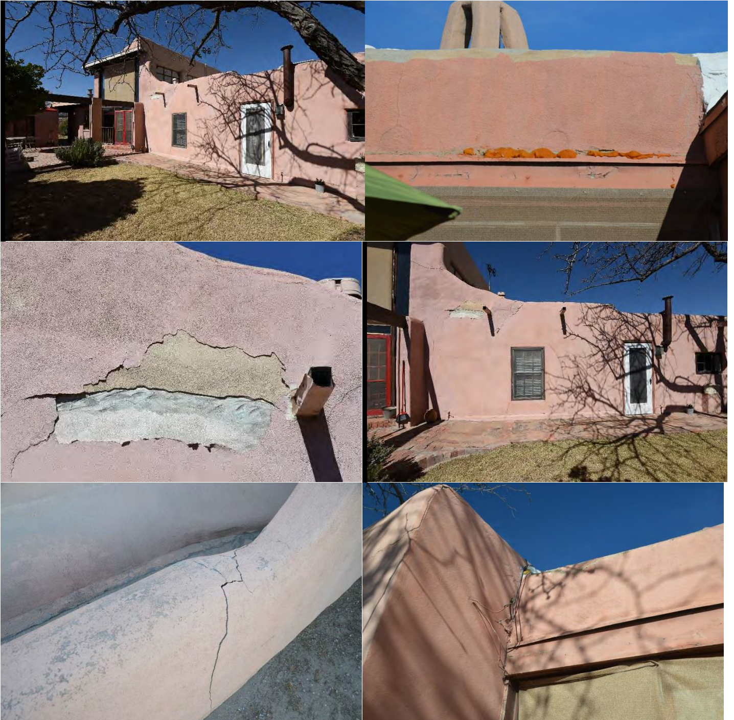
Photos: Examples of widespread exterior plaster issues
