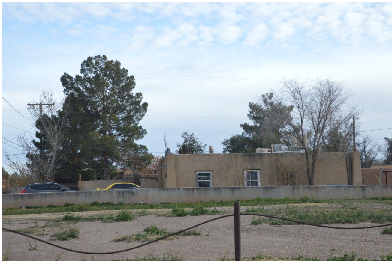
PHOTO OF NORTH SIDE OF DWELLING FROM CALLE DE CORREO SHOWING WINDOW TRIM TO BE PAINTED
