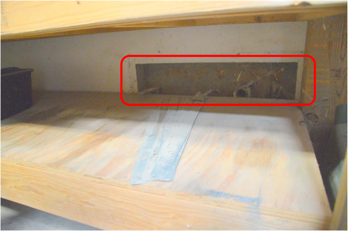
VIEW OF PLUMBING STUB-OUTS BELOW WORK BENCH
