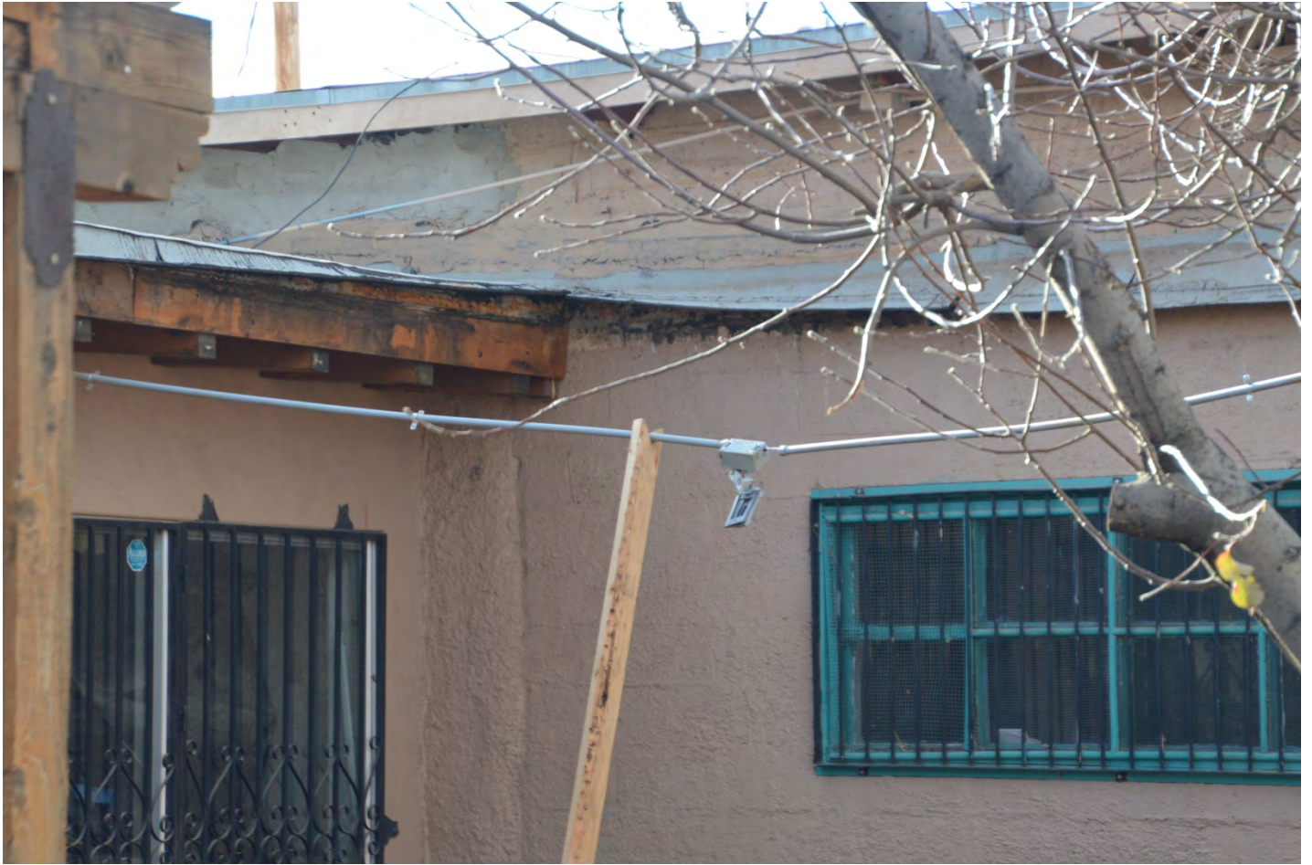
PHOTOS OF REAR OF DWELLING SHOWING HANGING ELECTRIC LINE (Taken 12/27/18)
